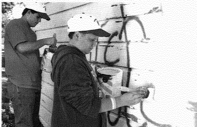
Graffiti needs to be cleaned up as soon as possible.
