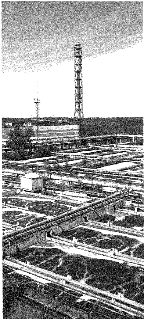
Water treatment facility
